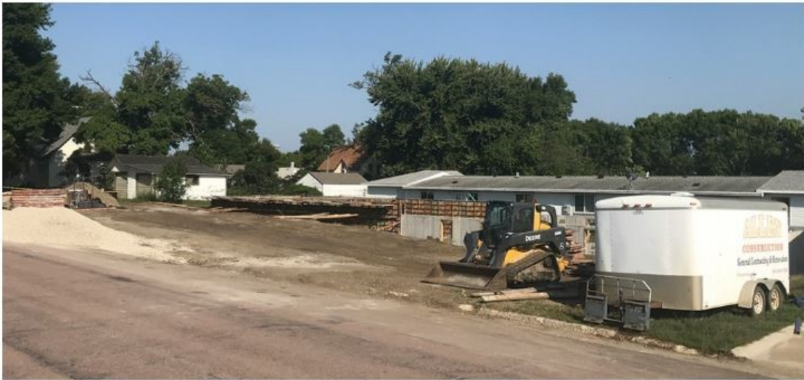
📷 An eight-plex being built on Broad Avenue has raised concerns from neighbors. A permit for the building was mistakenly issued by the city without considering zoning requirements.
